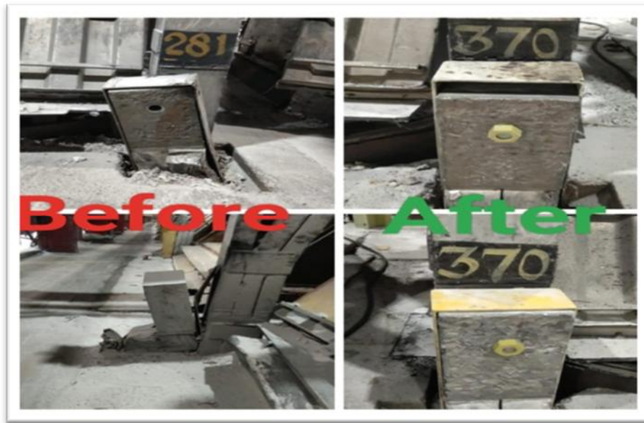
Figure 1. Sud bolt fixing for shunt alignment: before (left) and after alignment (right).
