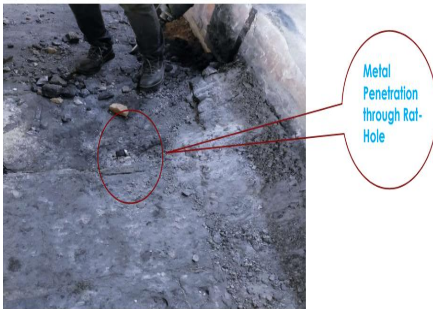
Figure 2. Rathole developed from cracks during power interruptions.
